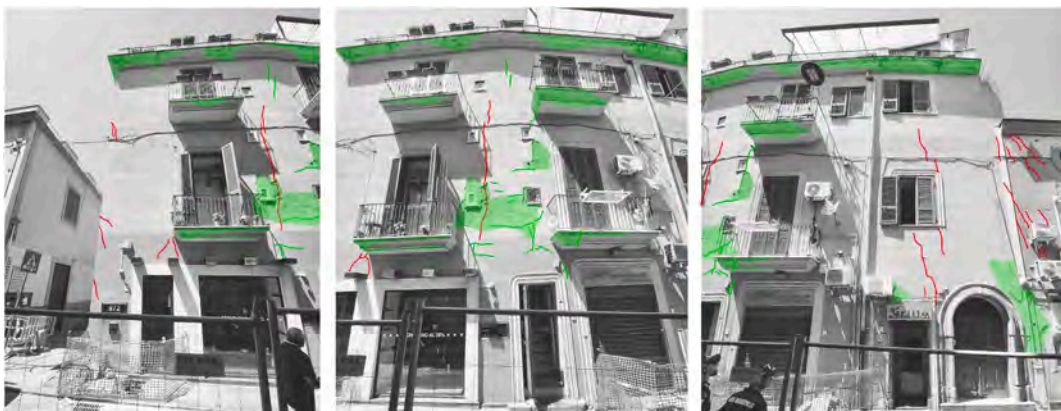
Fig. 3. Graphical representation of the crack patterns observed on the investigated façade and identification of the degradation and damage phenomena observed on the building envelope. In red are the anomalies clearly associated with the subsidence of the foundation soil; in green are the anomalies not directly attributable to the subsidence.
