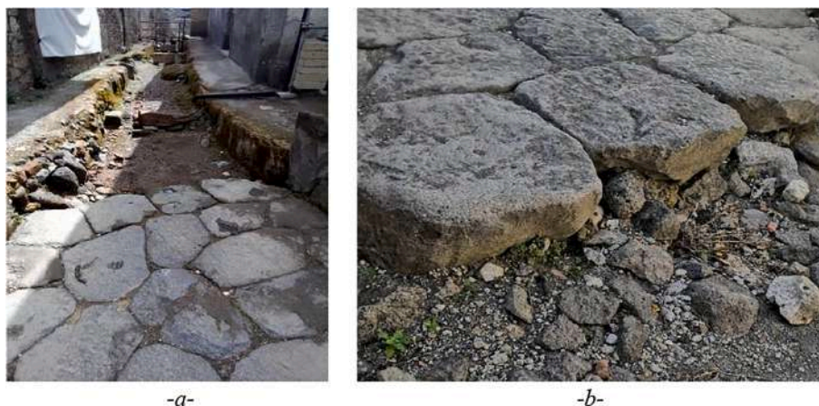
Fig. 3. Detail of the road section where paving work stopped at the moment of eruption: (a) Photo overviewing the alley, direction N—S; (b) Detail: photo of the section between the paved and the un-paved stretch of the alley.
