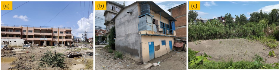
Fig. 18 (a) Functionality loss due to inundation and debris deposition in RC building, (b) an example of flood damaged semi-permanent building along the Manohara corridor, (c) damaged corn field by the 2024 flood
