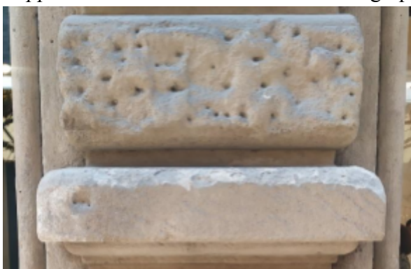
Fig. 1: The Bossage under study with evident damage due to flaking and exfoliation. Samples are taken from areas already decoached without further damage to the artwork
