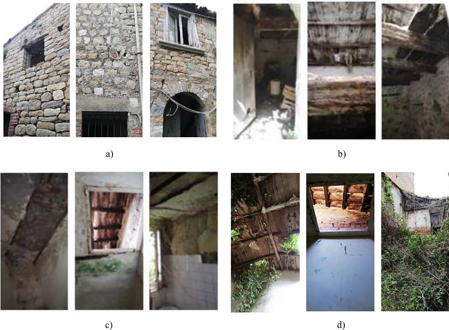
Fig. 3 Photographic documentation of the crack pattern: (a) Crushing phenomena of vertical masonry walls; (b) Degraded wooden beams; (c) Corrosion phenomena on steel beams; (d) Collapse of the roof of SU7
