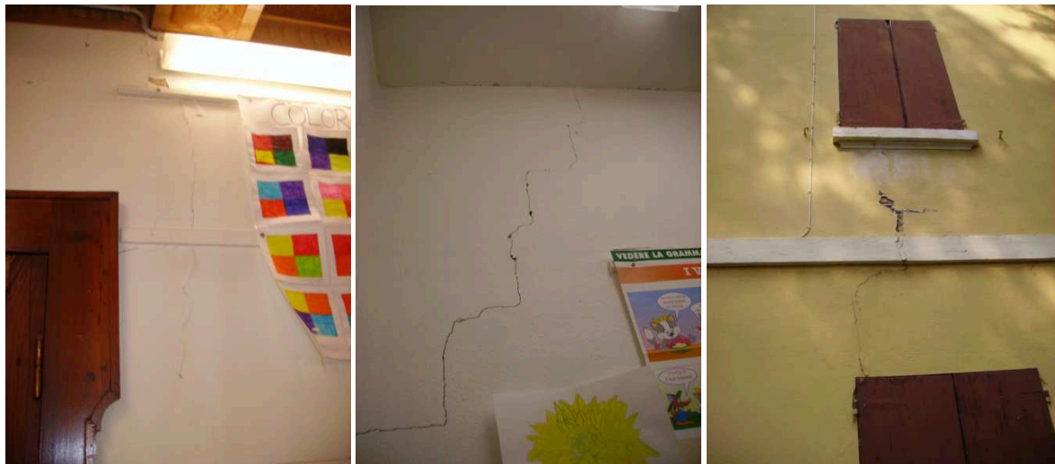
Fig. 4. Details of some internal and external cracks
