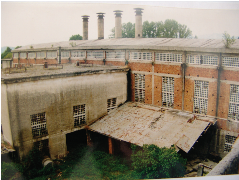
Fig. 17. Local view of boilers. Paper Mill of Atina. Municipal Library of Atina..
