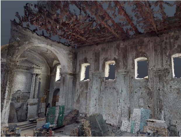
Figure 6: Indoor view of the Matterport Pro2 3D's point cloud: note, in particular, the covering
