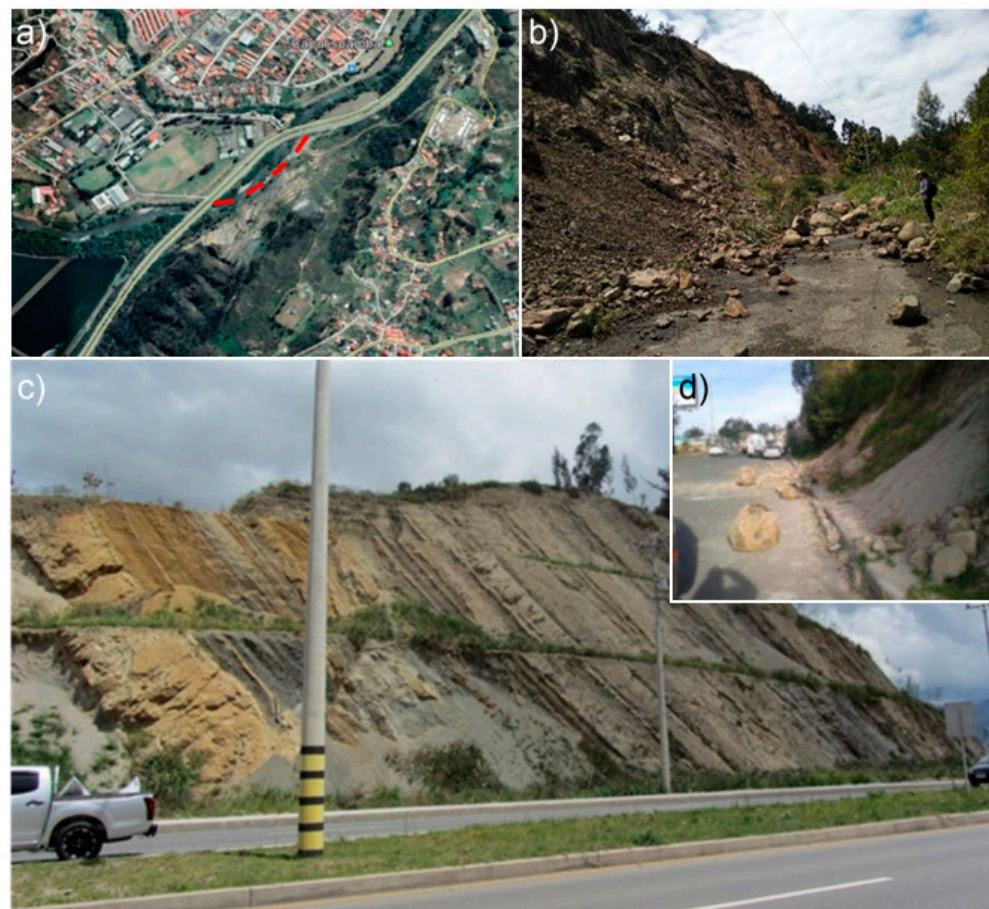
Figure 2. The functionality of the Pan-American Highway is often interrupted by rockfalls. (a) Deviation of the original road axis (red dotted line) caused by rockfall events; (b) landslide deposits have almost completely invaded the highway; (c) over-dip cataclinal slope: the stratification is slope-oriented; (d) boulders detached from the slopes block the lane.
