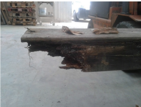
Fig. 7 – Degradation of the beam on bearing
